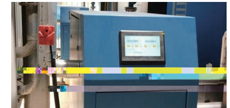
Waste Heat Recovery Transformation of Air Compressor
